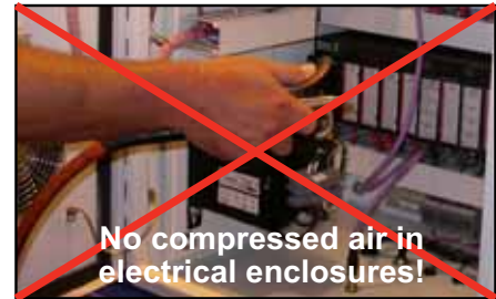
Figure 7-1: Never Use Compressed Air Inside an Electrical Enclosure
